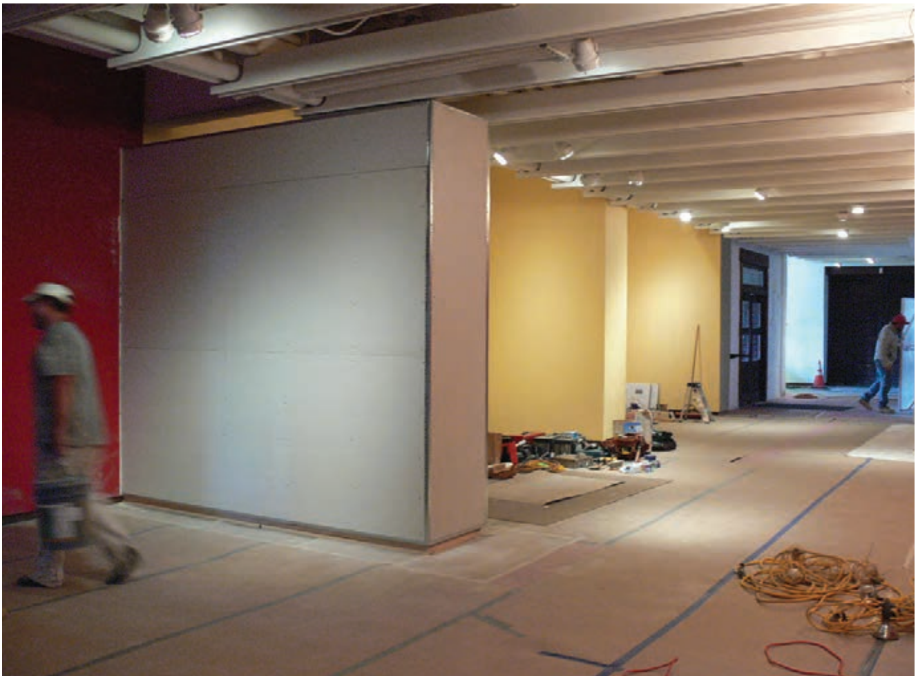
The Goodwin Gallery during the renovation process. The newly uncovered windows at the far end shed light on the entrance to St. Francis Auditorium. Photograph by Michelle Gallagher Roberts.
